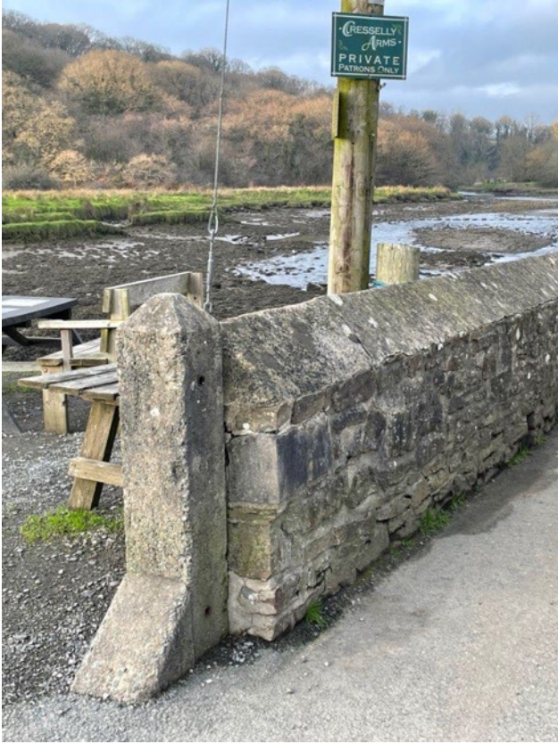
Figure 24: Photograph showing an example of sloping rendered copings to stone walls around the village.
