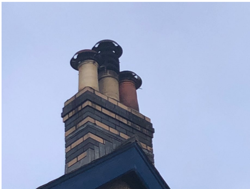
Figure 21: Photograph showing a colourful buff and blue brick chimney to the Manse.
